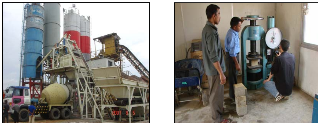
Fig-12: Concrete batching plant and material testing facility at Third Karnaphuli Bridge site
