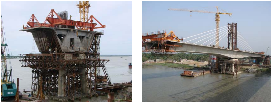
Fig-16: The balanced cantilever method of construction was used for Third Karnaphuli Bridge
