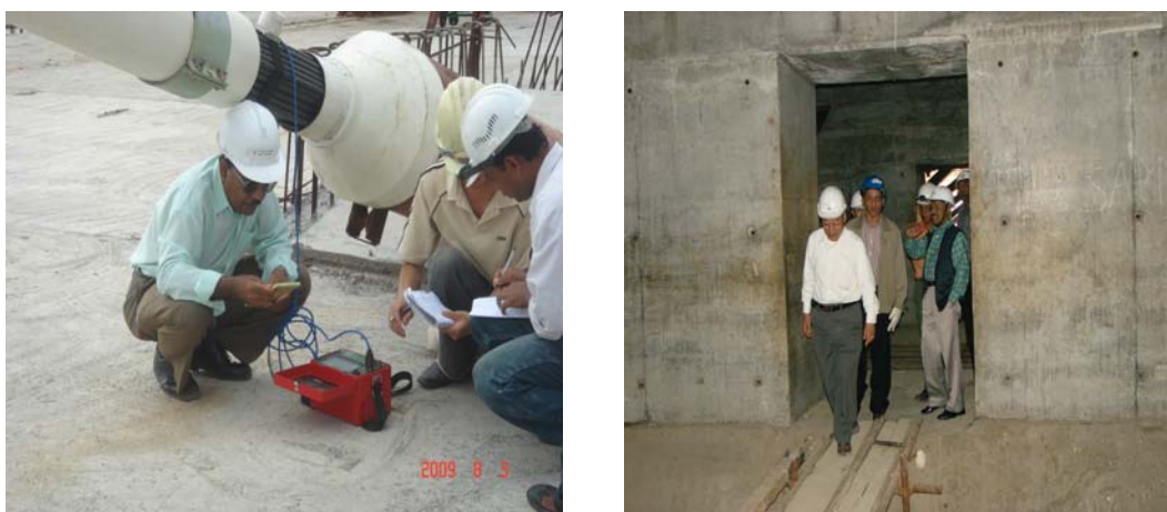
Fig-17: Measuring of stress level at stay cable in progress and access inside the bridge deck
