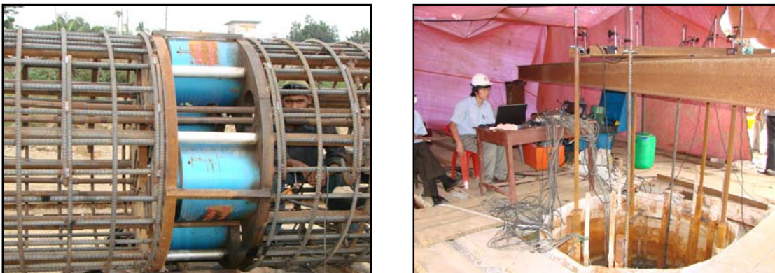
Fig-5: Arrangement of Load Cell in Rebar Cage and Progress of O-cell Pile Load Test
