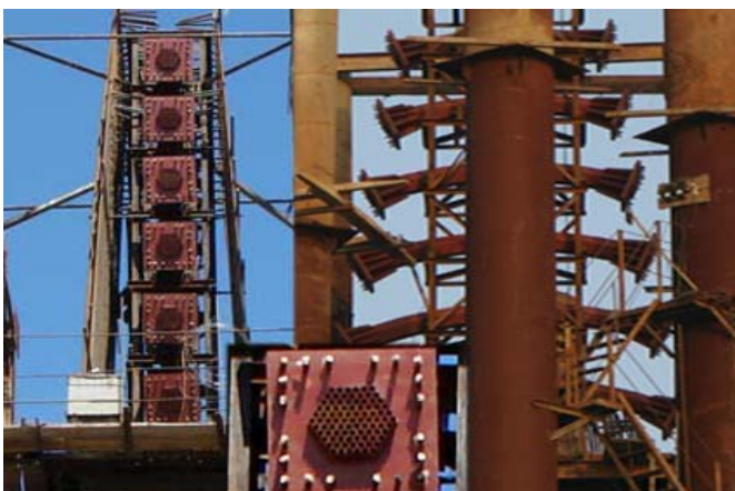
Fig-10: Damper anchorage system of stay cable finished tower with stay cable and saddle of Third Karnaphuli Bridge
