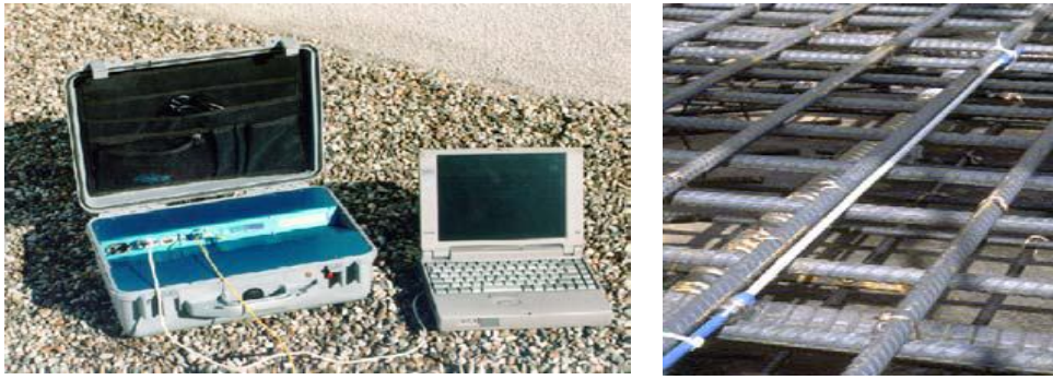
Figure 7. SOFO system reading unit & sensor installation (Inaudi, 2005)
