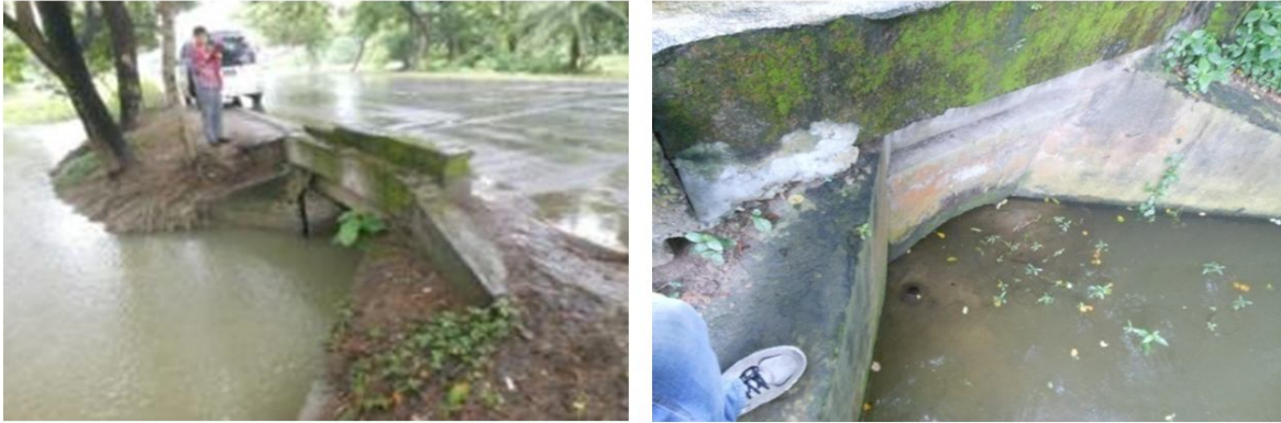
Figure 4. Deteriorated structural condition in (a) Slab Culvert at chainage 211+018 and in (b) Arch Masonry at chainage 5+028
