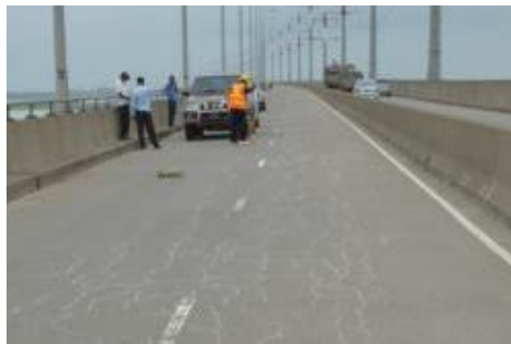
Figure 2. Longitudinal cracks upon bridge deck-overhang
