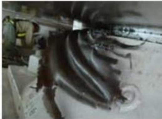
Picture1. Damage of Movable Bearing
