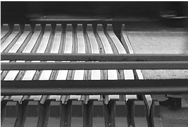
Figure 2. Existing Modular joint in distressed condition
