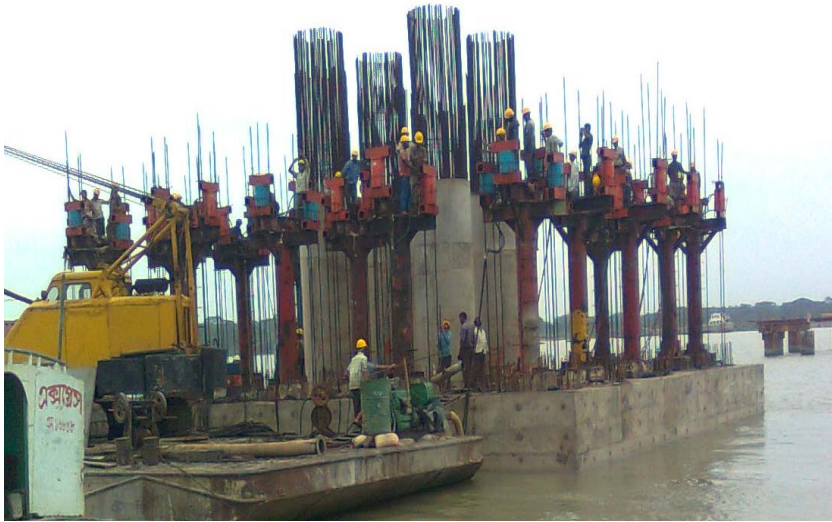
Figure 3: Lower of pile cap in progress through precise synchronized operation of hydraulic jacks
