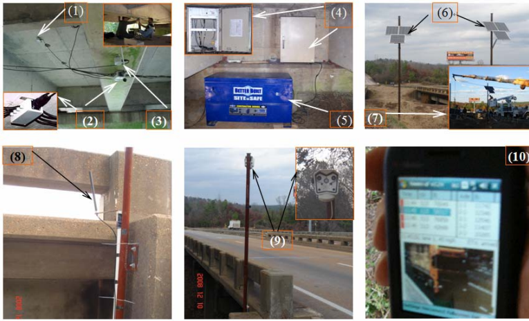
(1) FAD sensors; (2) Spider; (3) Weighing sensors; (4) Cabinet & panel; (5) Batteries housing; (6) Solar panels; (7) Solar panel installation; (8) Antenna; (9) Camera; (10) PDA
