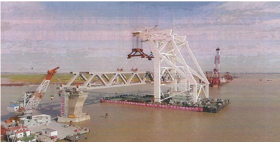
Figure 13. Erection of fabricated 3088 metric ton fabricated truss on two adjacent piers by 4000 metric ton capacity barge mounted crane.
