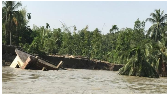
Figure 7. Erosion at Naria, few km downstream of Padma Bridge.
