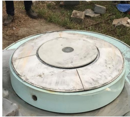
Figure 5. Friction pendulum bearing (cover removed for inspection).
